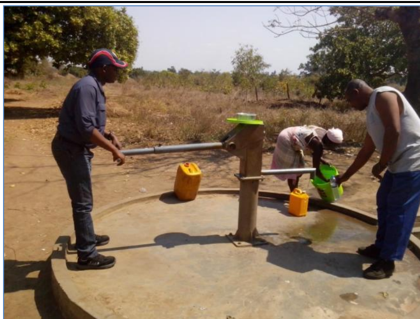
Figure 4.19 Drinking Water Well
