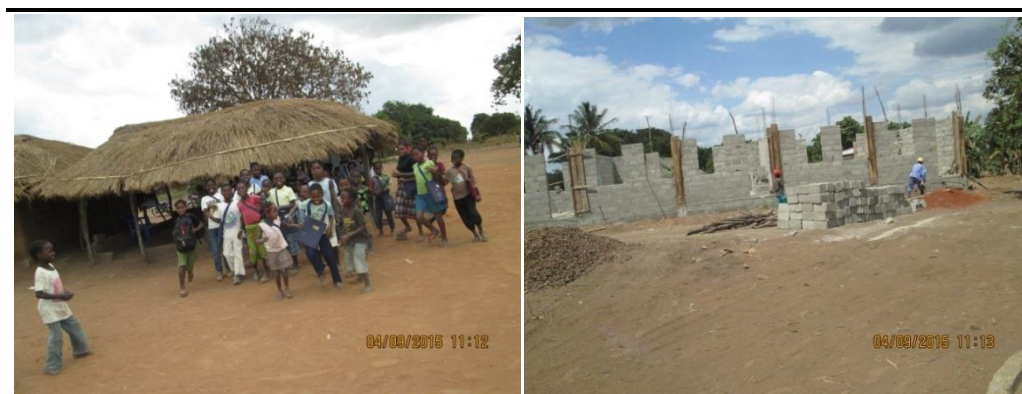
Figure 4.30 Present Primary School of EP1 and of EPC under Construction in Bairro de Mugonda
