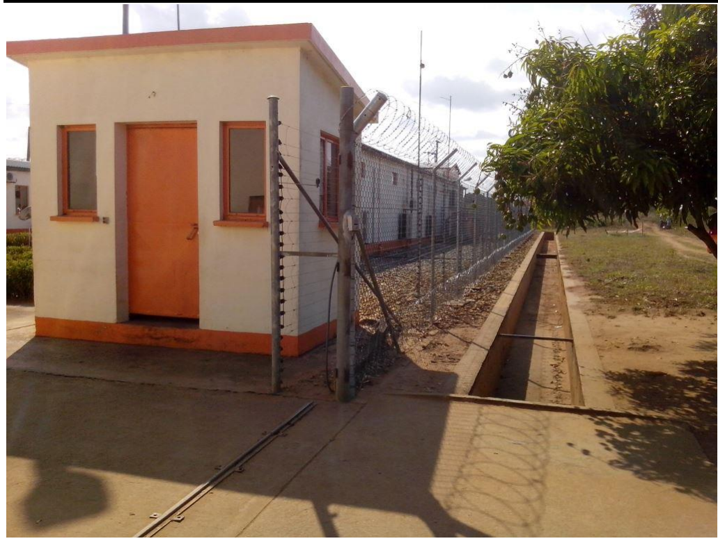
Figure 4.22 Substation of Mocuba
